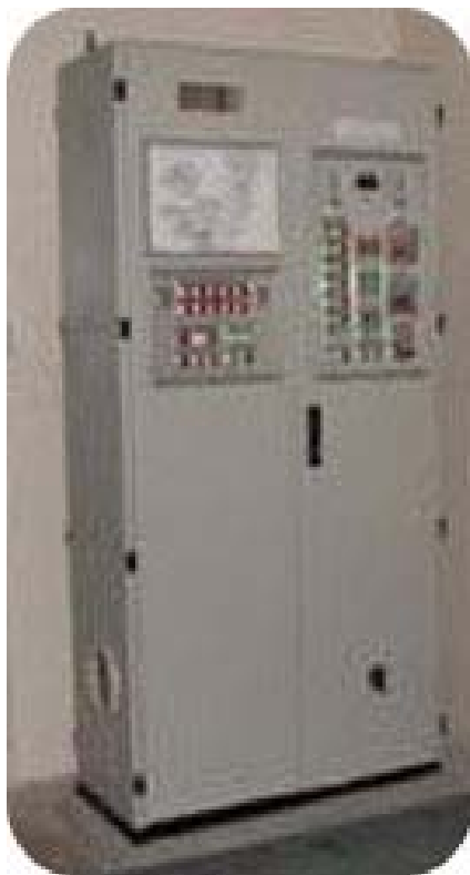
Fig.1 : Electrical Control Panel
